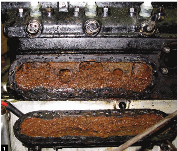
1 The rear side plate on the block was removed and revealed rust and silt build-up that significantly occluded water circulation and cooling in the block.
